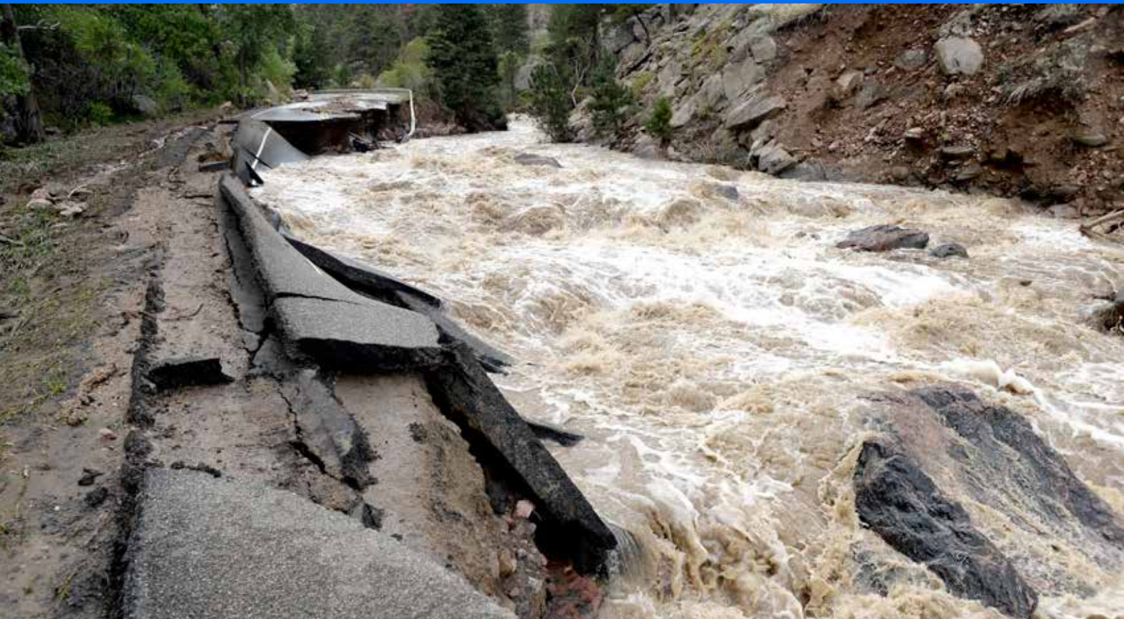
Damage to Lefthand Canyon near Boulder, Colorado from September 2013 floods. Photo: Jeremy Papasso/AP.
