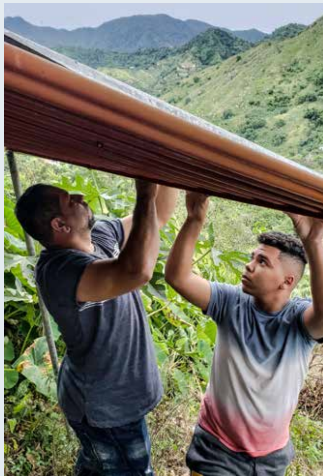
Father and son installing a water collection system, using their own knowledge and materials. Jayuya, Puerto Rico. Photo: Fernando Briones.
