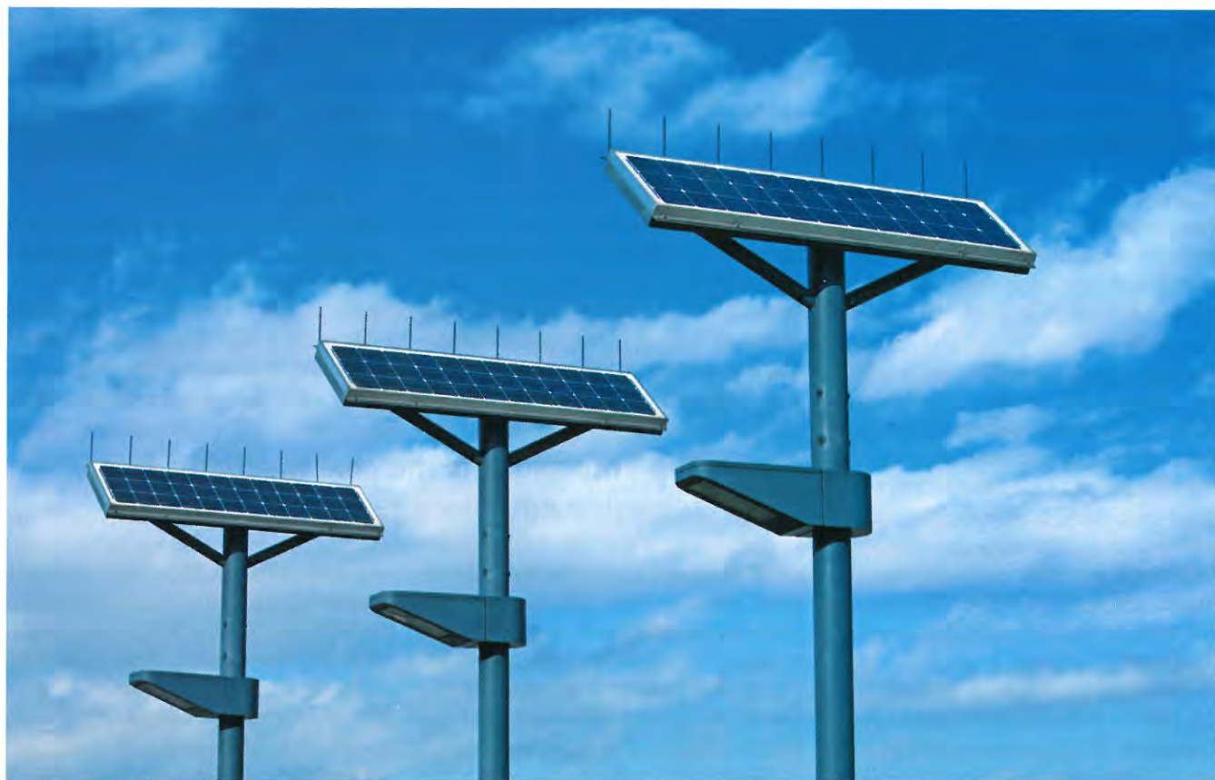
Solar powered street lamps, Yokohama, Japan.
