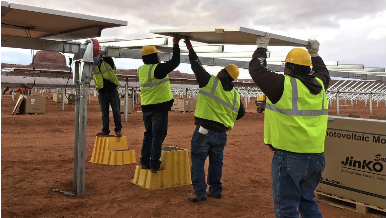
The construction project to build the Kayenta solar farms on the Navajo Nation, shown here in 2018, employed hundreds of people, nearly 90 percent of whom were Navajo citizens. Photo: Navajo Tribal Utility Authority / Navajo Nation.
