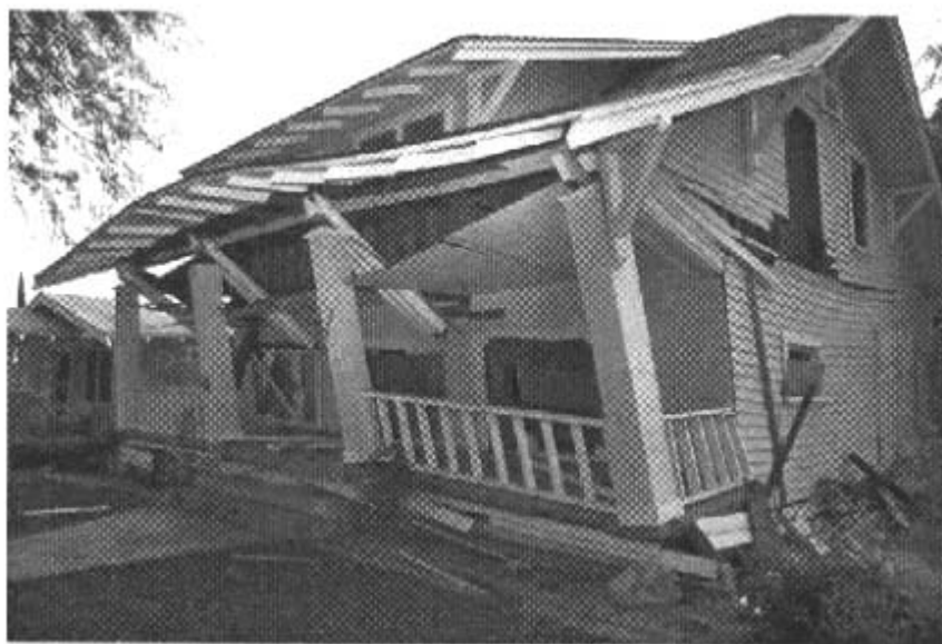
Residential destruction resulting from the Northridge, California earthquake in 1994. (Photo courtesy of FEMA.)
